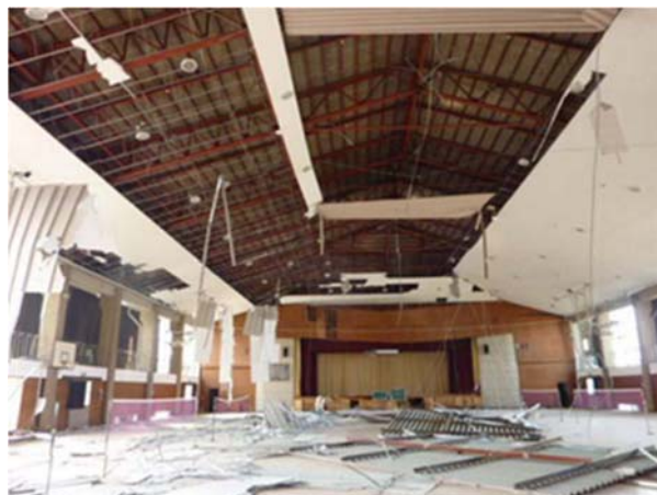
Figure 1: Ceiling collapse that occurred during the 2011 Great East Japan Earthquake 1
