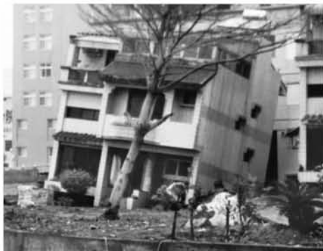
Fig. 5 A house tilted due to liquefaction of the supporting ground (Jiji earthquake, Taiwan, 1999).
