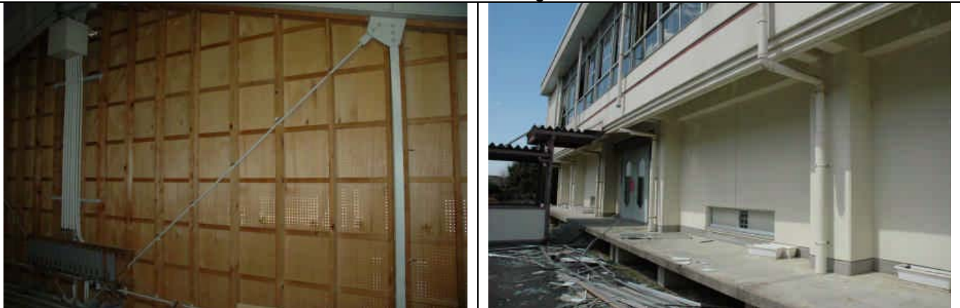
Photo 11: Vertical brace members in the end wall and first-story reinforced concrete column were undamaged.
