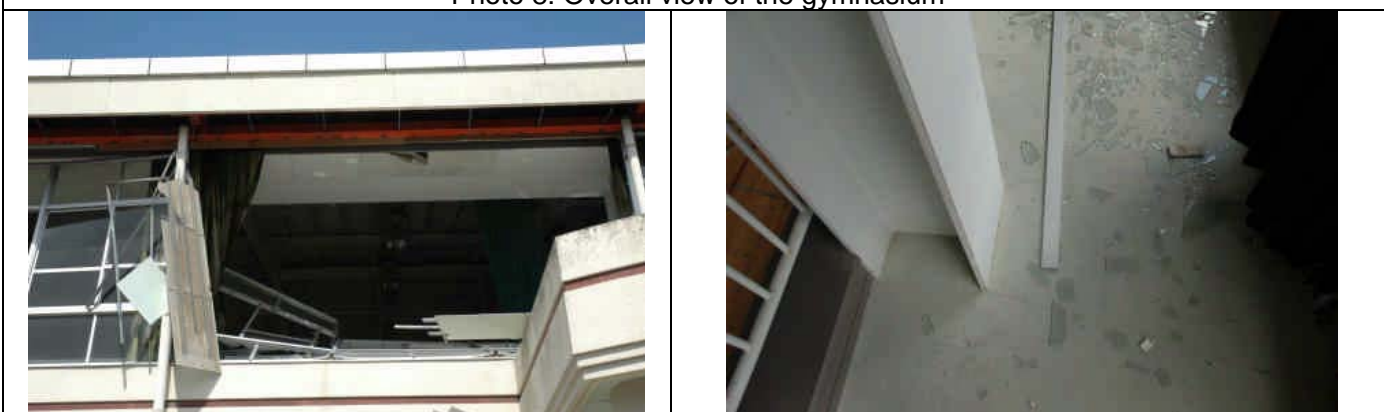
Photo 9: Fall of glass panes and cracking at the base of a steel column
