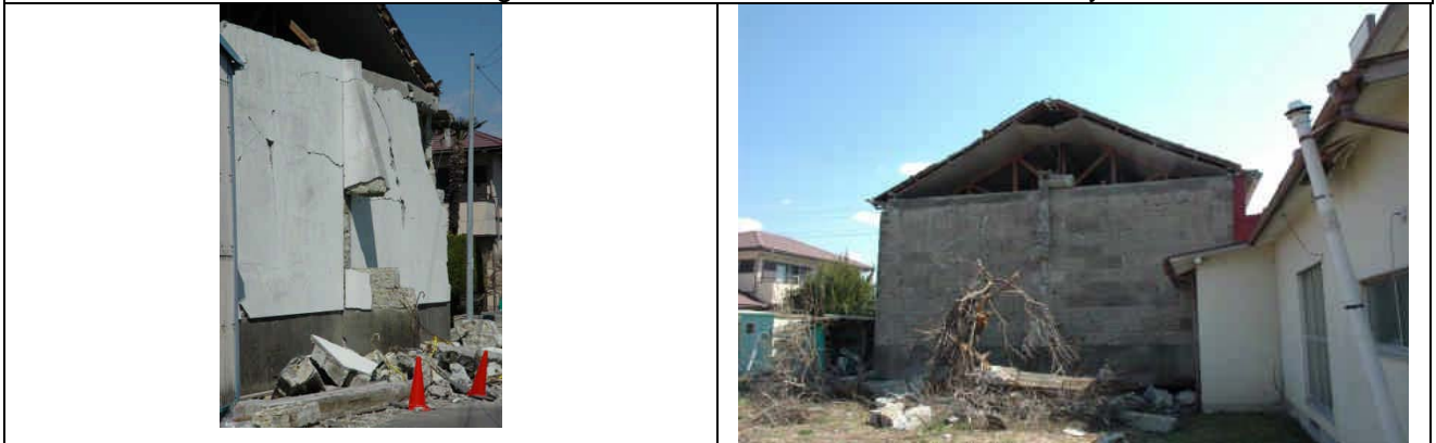
Photo 3: Damage of Masonry Warehouses near Gundo Elementary School
