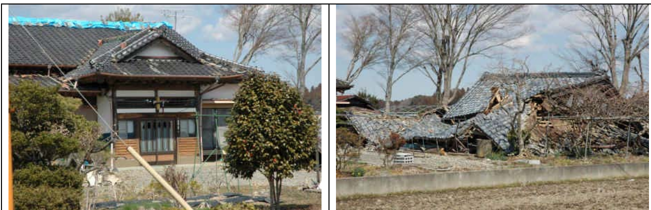
Photo 7: Fall of exterior wall finishing of a house and collapse of a timber traditional barn
