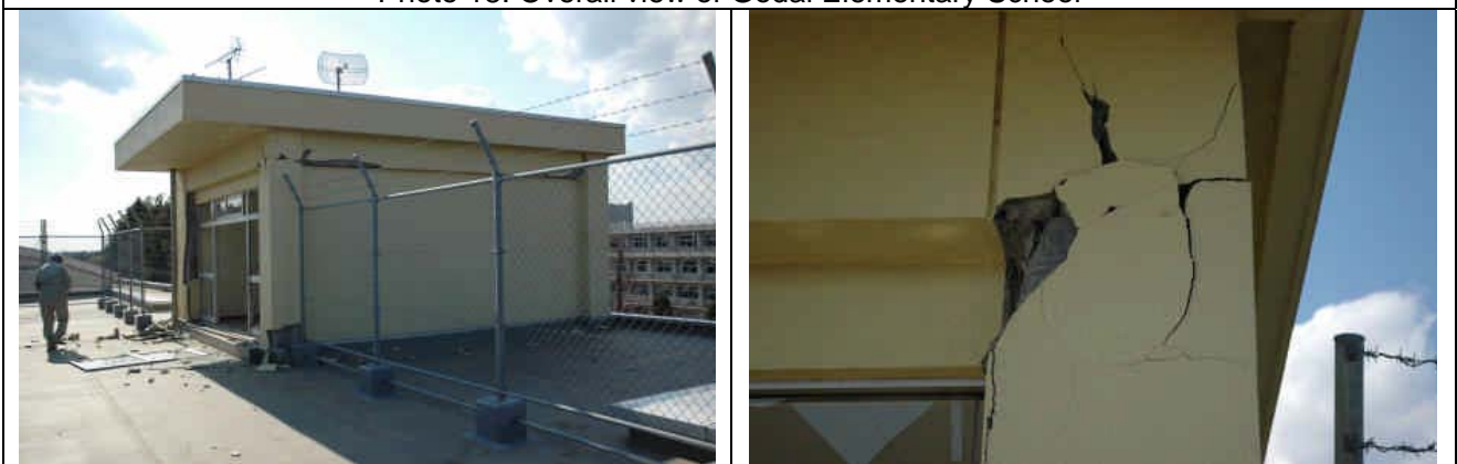
Photo 19: Damage of the penthouse
