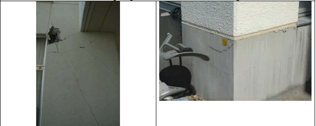
Photo 14: Diagonal crack at the top and crack at the base of a first-story column
