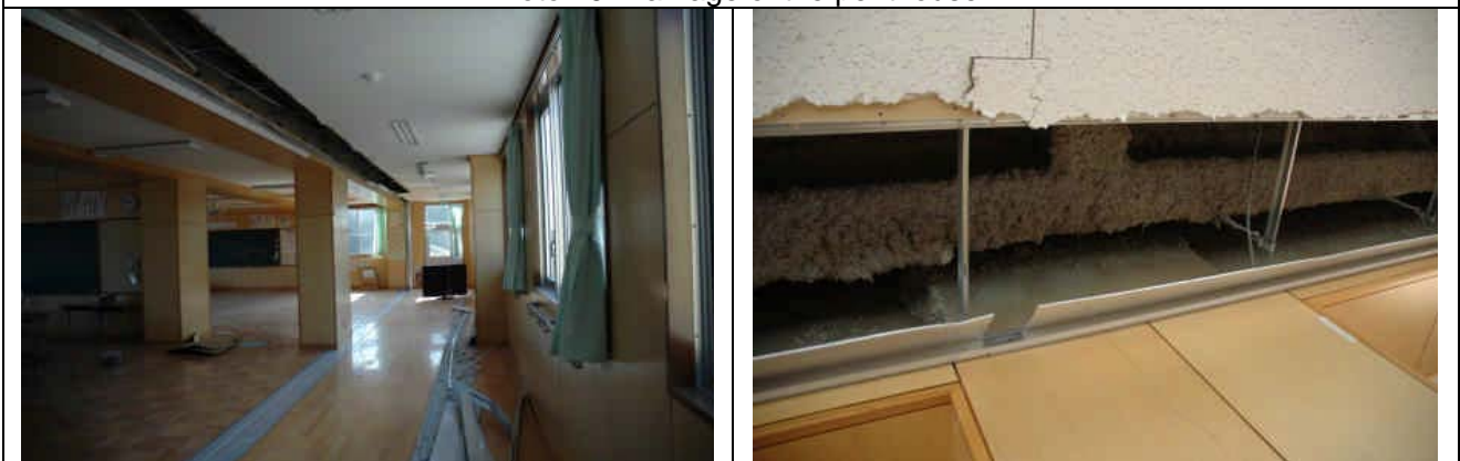
Photo 20: Damage of expansion joint between the existing and a new addition
