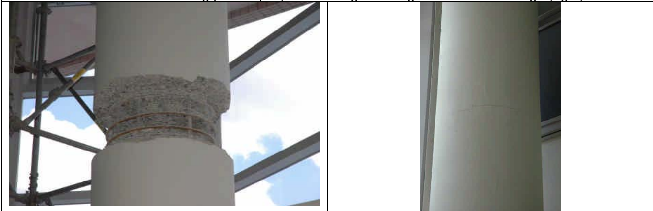
Photo 17: Damage of tall columns in the entrance hall
