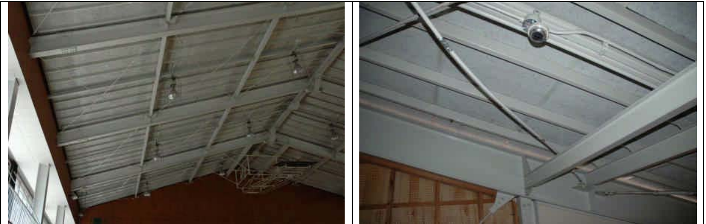
Photo 10: Deformation of ceiling brace members
