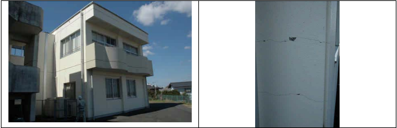
Photo 1: Flexural cracks in columns in a building in accordance with the New Seismic Design Provisions
